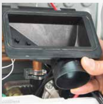
Inspection of condensates tray
