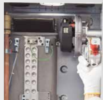
Opening of the complete combustion system
