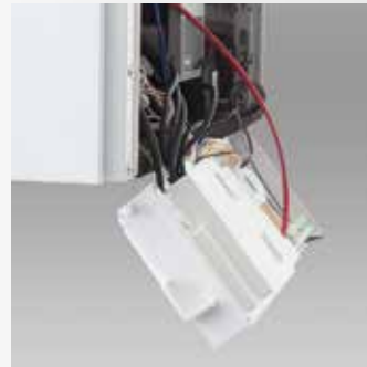
Opening of the panel board.
